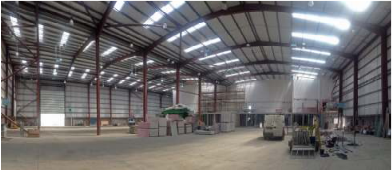
Internal Panoramic View of Main Working Floor, including construction of mezzanine floor
