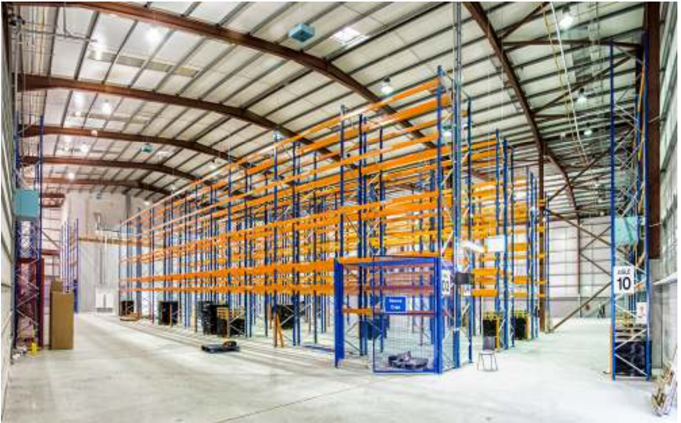
Newly installed High level Eurotech racking system on factory floor, requiring super-flat floor surface
