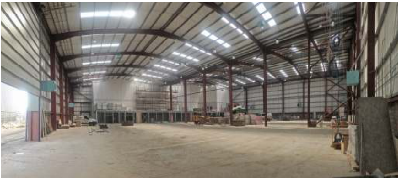
Internal Panoramic View of Main Working Floor, including construction of mezzanine floor
