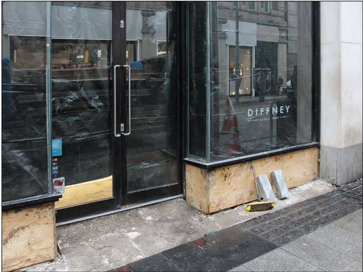
New stone plinth required to existing Shopfront
