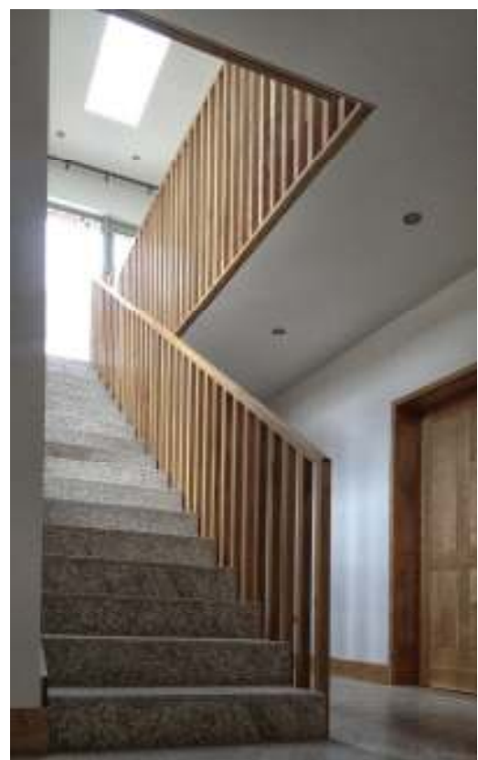
Bespoke oak timber handrail
