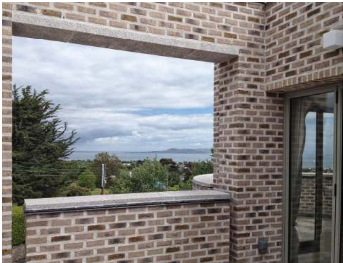
2 nd floor balcony, with suspended granite capping. Slate and lead roll drip under granite capping
