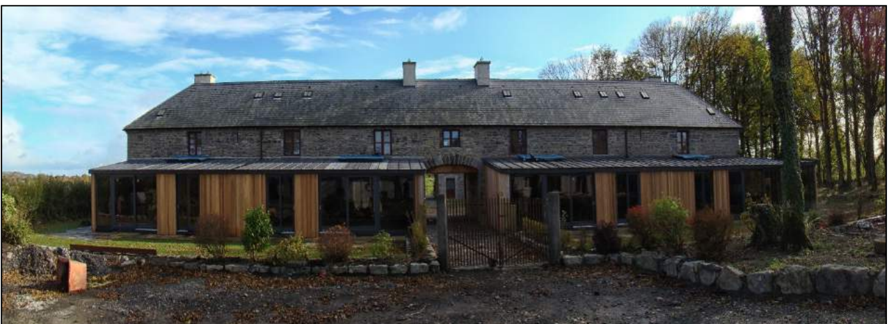
Rear extension to Clonabreany Courtyard, including timber external cladding, zinc-clad flat floors and alu-clad sliding doors and windows
